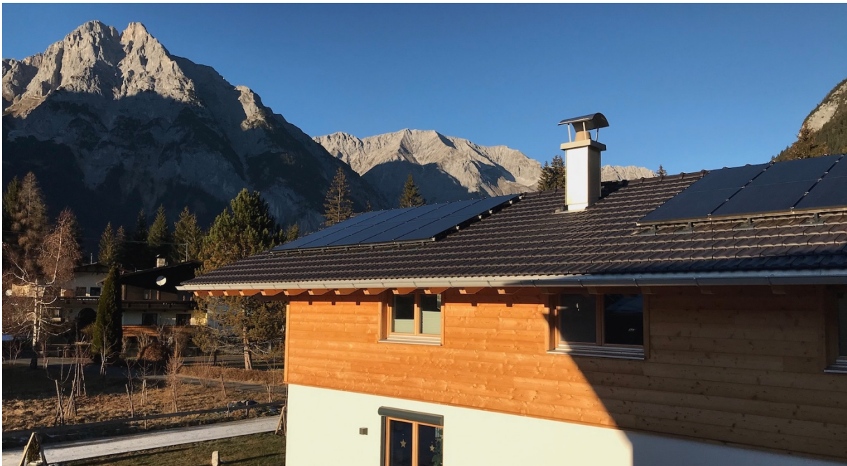
Photovoltaik-Anlage in Leutasch, © Marlene Buchinger
